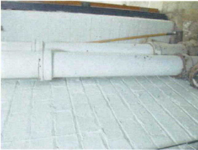
Exposed Waste Pipe in Boiler Room
