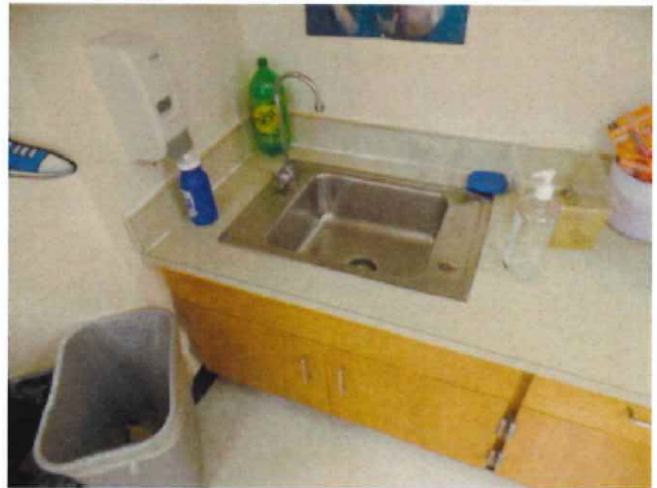
Classroom sink without fountain
