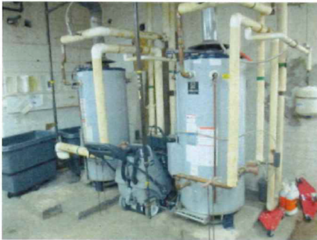
Domestic Hot Water Heaters
