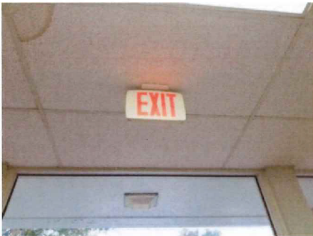
Noncompliant Exit Sign
