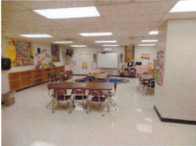
Fluorescent tubes to be removed
