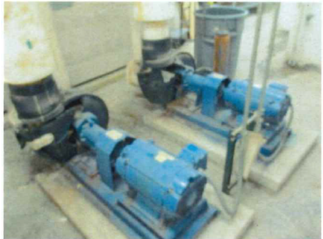
Heating Hot Water Pumps
