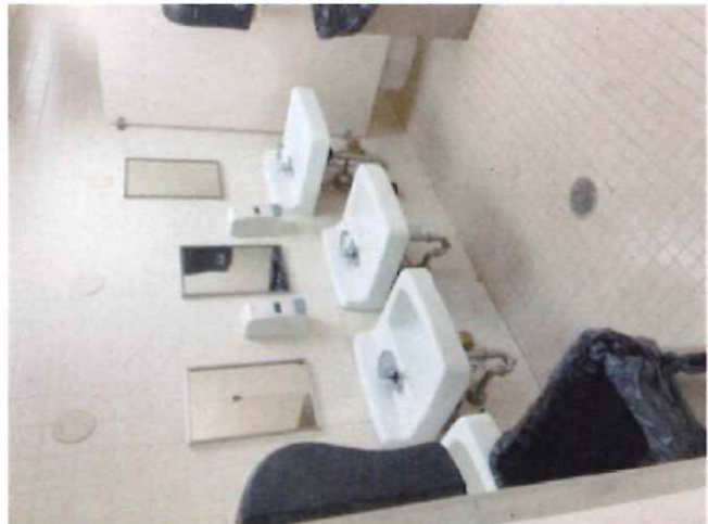
Non-compliant fixtures and mirrors
