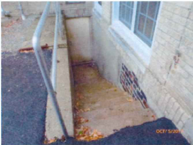
Stairwell missing handrails
