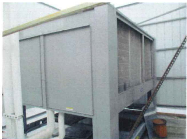
Air Cooled Condenser
