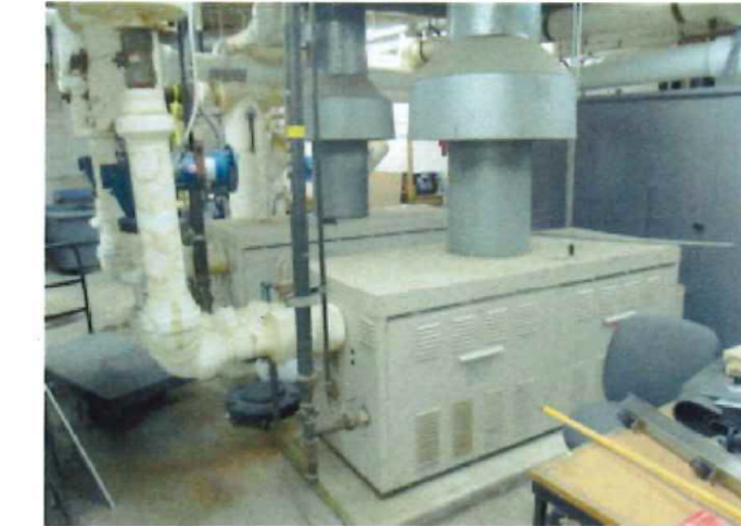
Gas Fired Boilers
