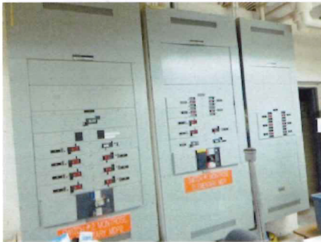
Main Distribution Panelboards
