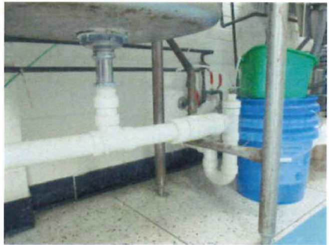
Kitchen Sink Waste
