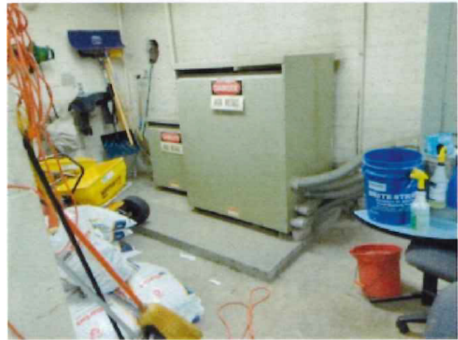
Indoor Utility Transformers
