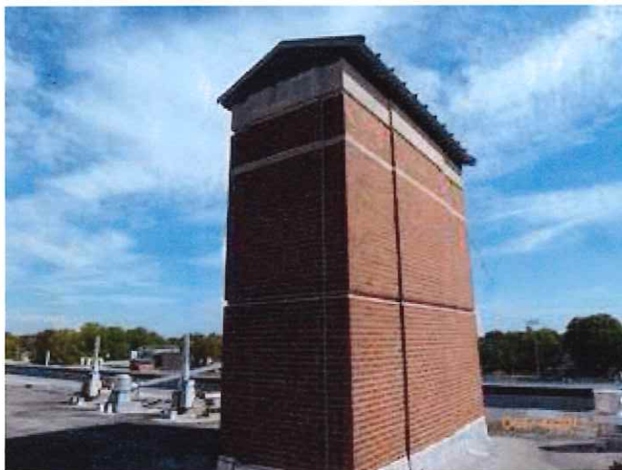
chimney to be tuckpointed
