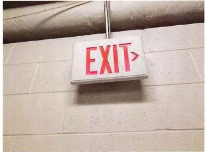
Noncompliant Exit Sign
