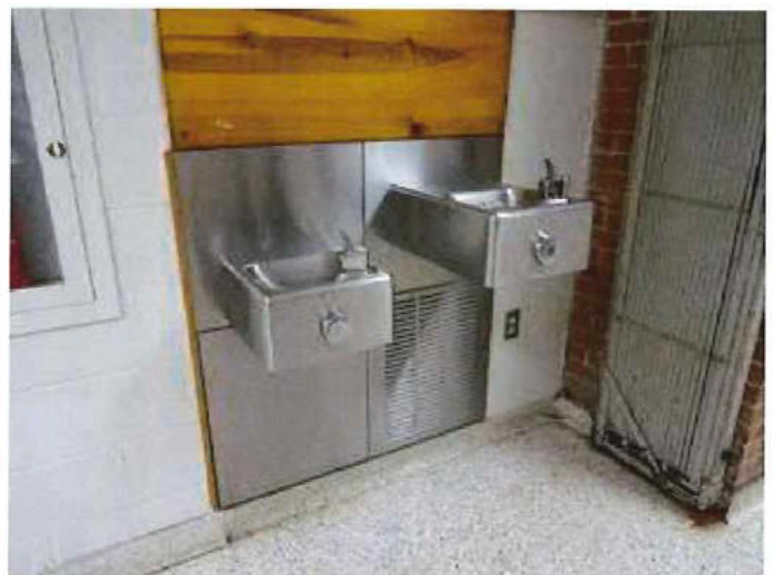
ADA Electric Water Coolers
