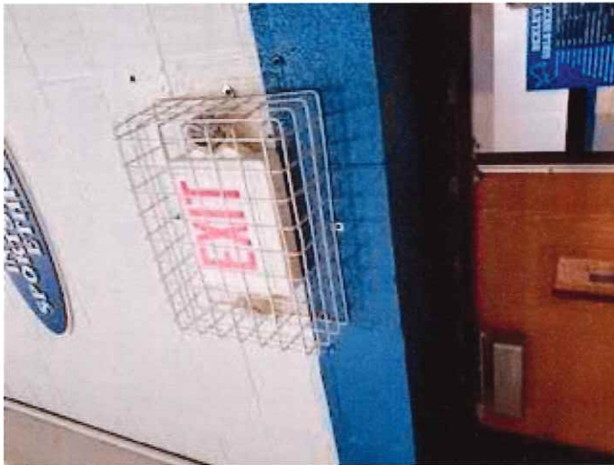
Gymnasium Exit Sign with Egress Floods
