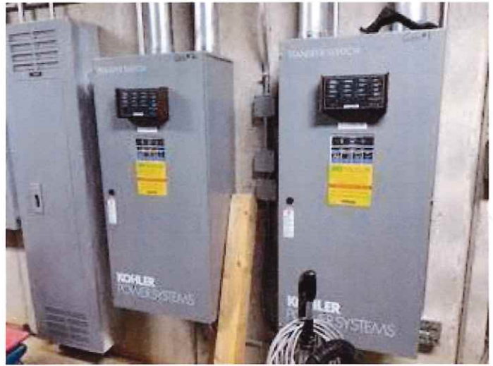
Facility Transfer Switches
