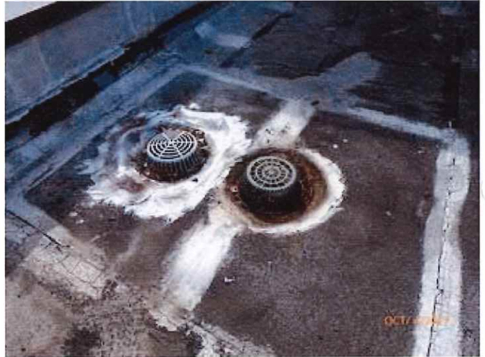
Roof drain and overflow drain
