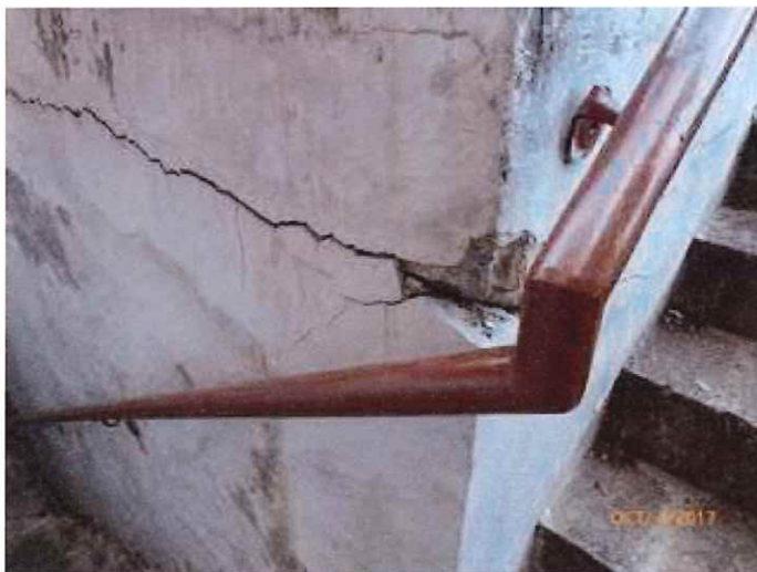
Stairwell that needs repaired
