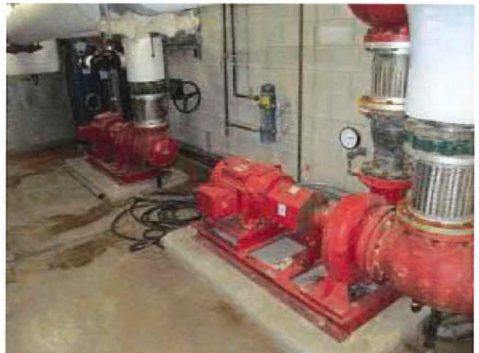
Heating Hot Water Pumps
