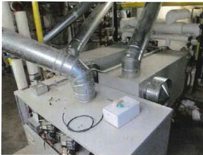
Gas Fired Water Heater
