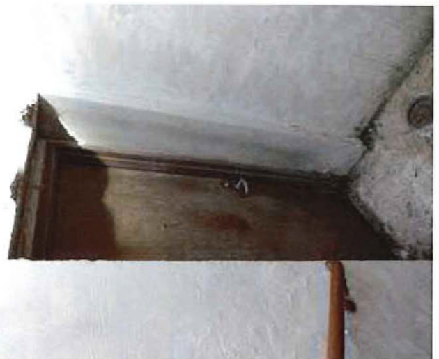
Exterior door to be replaced
