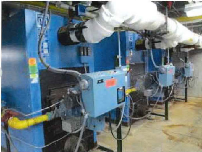
Gas Fired Boilers
