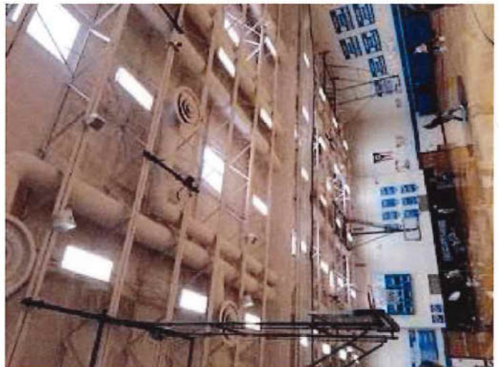
High School Gymnasium Lighting
