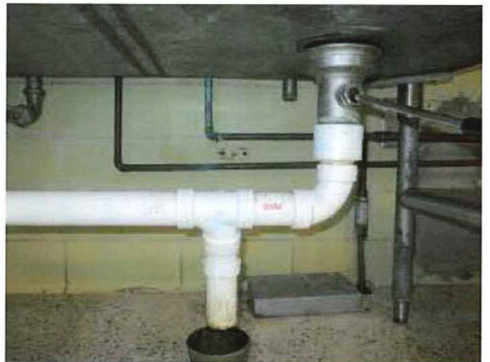
Kitchen Sink Waste
