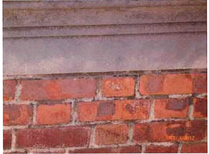
Brick wall to be tuck pointed
