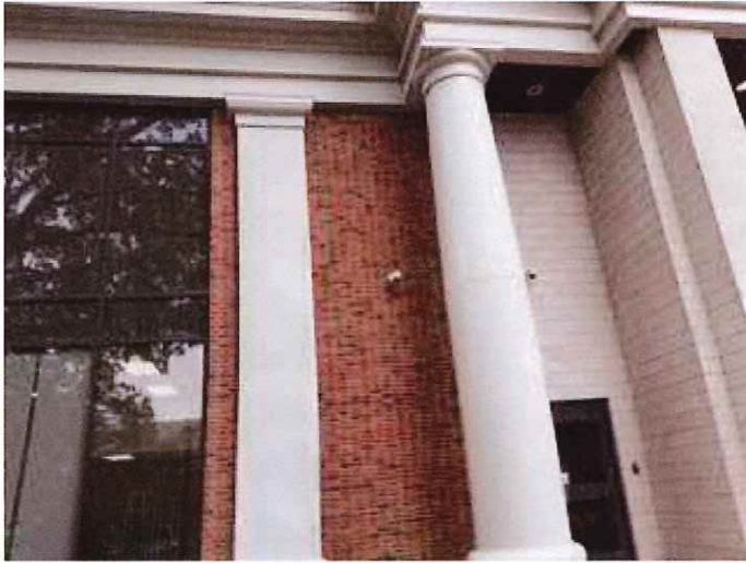
Exterior CCTV Cameras
