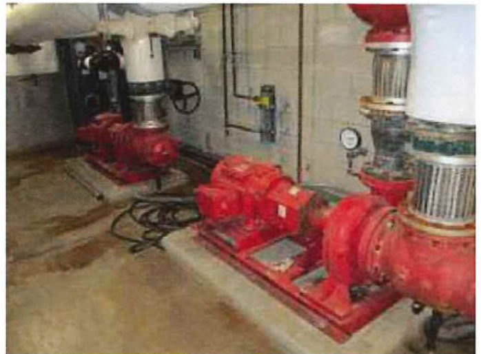
Heating Hot Water Pumps
