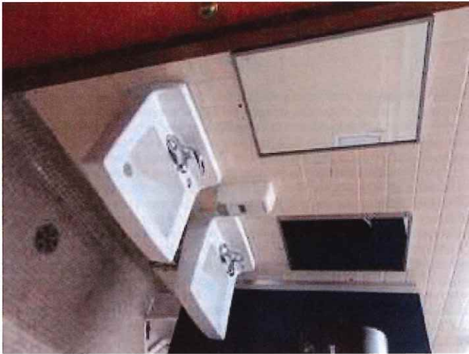
Non-compliant fixtures and mirrors
