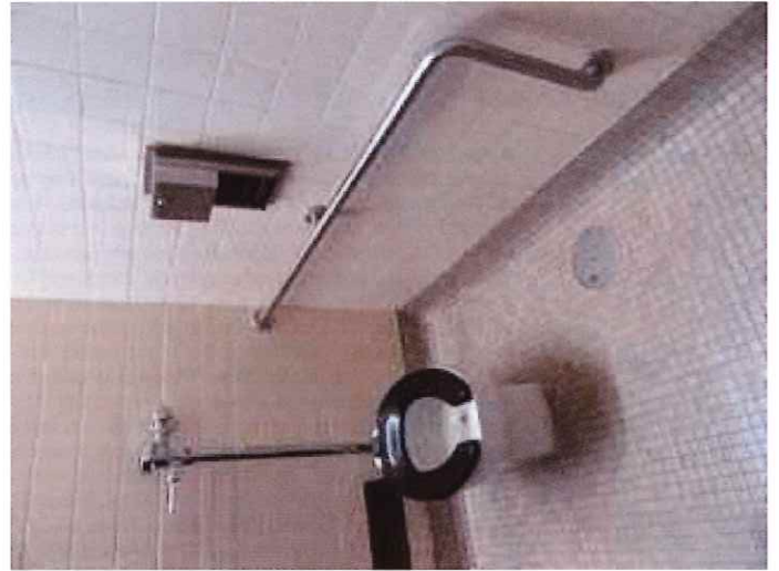
Non-compliant toilet accessories
