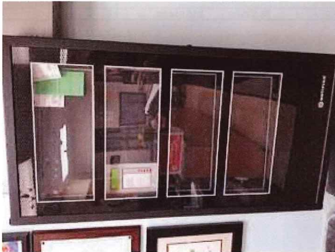
Fire Alarm Control Panel
