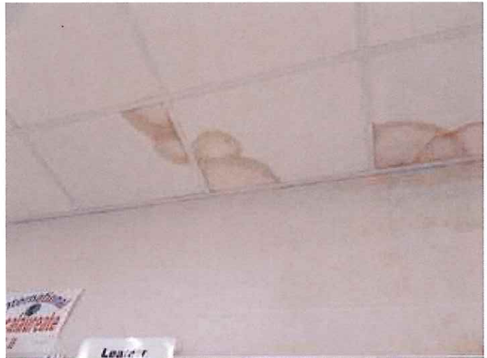
Damaged ceiling tile
