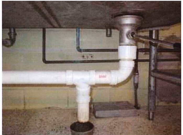
Kitchen Sink Waste
