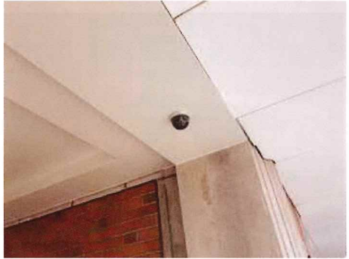
Interior CCTV Camera
