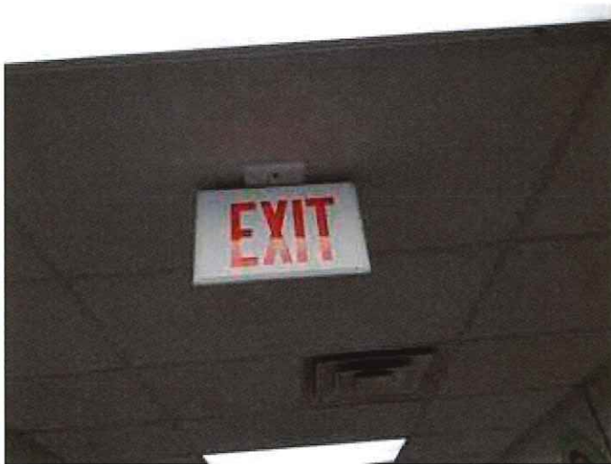
Noncompliant Exit Sign
