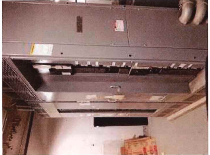
Elementary School Subdistribution
