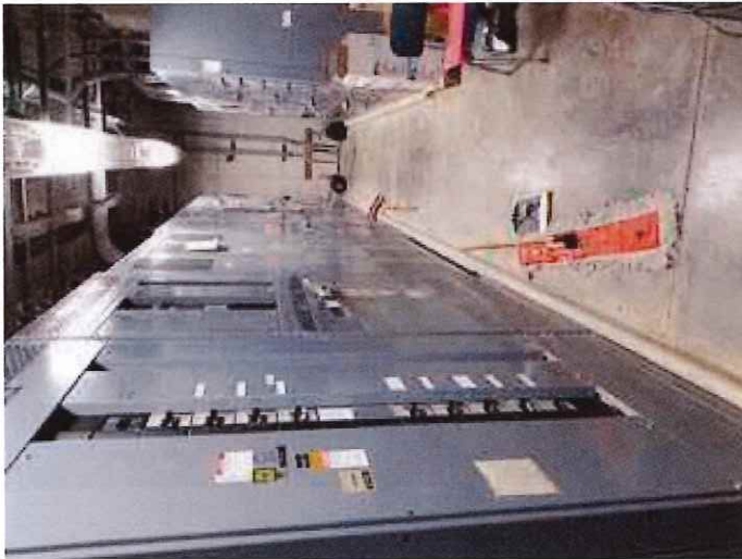
Main Distribution Switchgear
