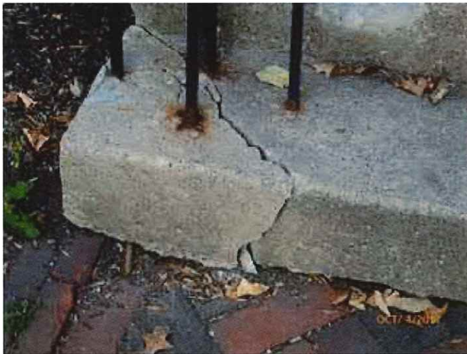
Broken concrete steps
