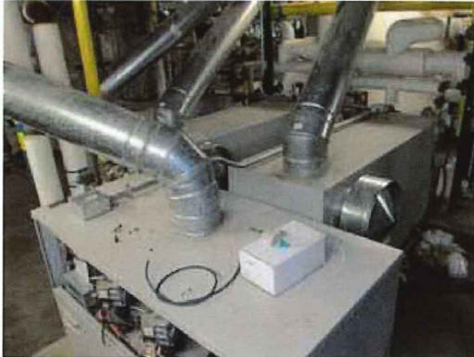
Gas Fired Water Heater
