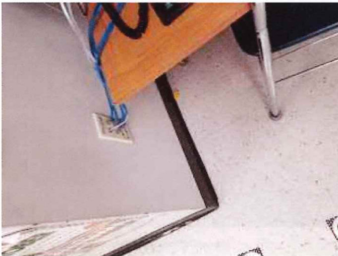
Typical Classroom Data Jacks
