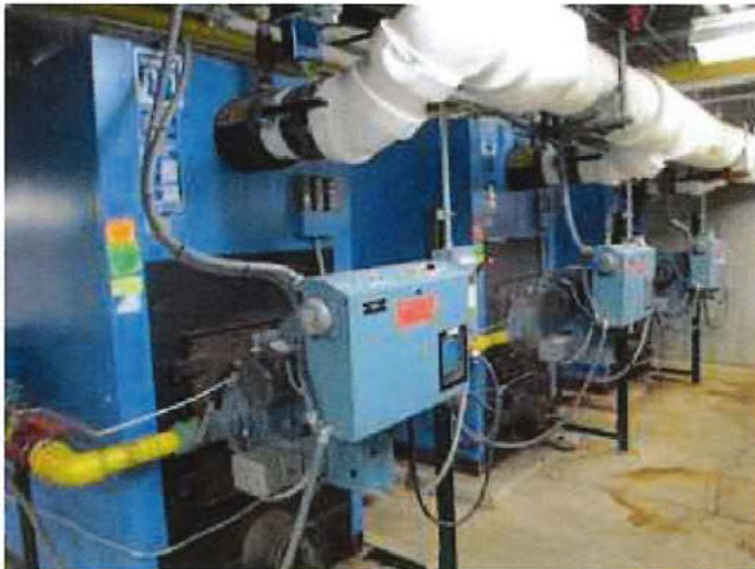
Gas Fired Boilers
