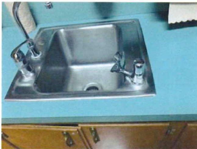
Non-compliant sink mounted drinking fountain
