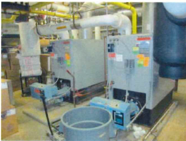
Gas Fired Boilers
