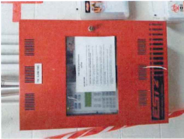
Fire Alarm Control Panel
