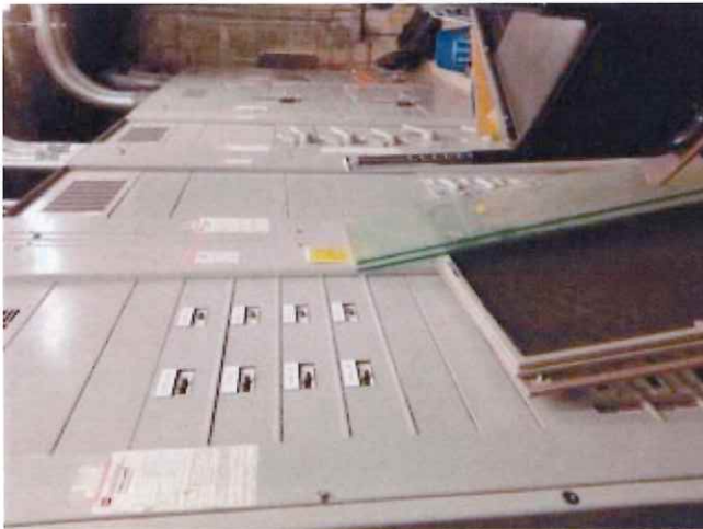
Main Distribution Switchgear
