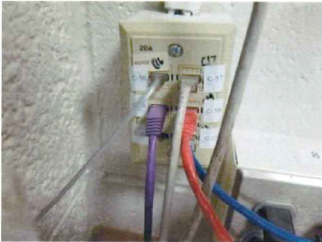
Typical Classroom Data Jacks
