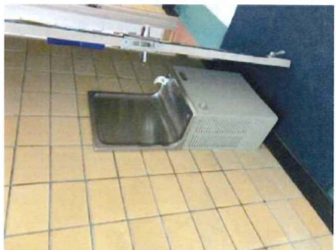
Non-compliant electric water cooler
