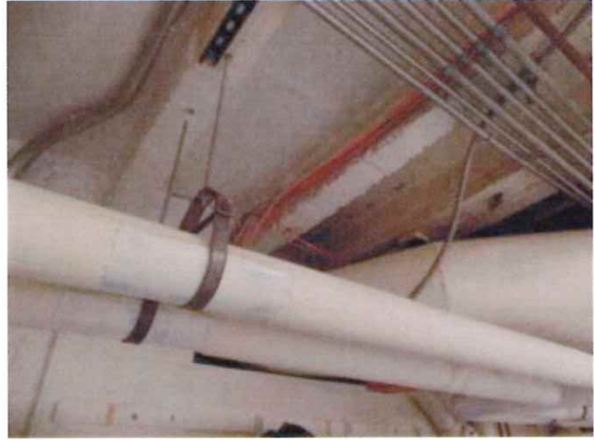
Asbestos free pipe insulation
