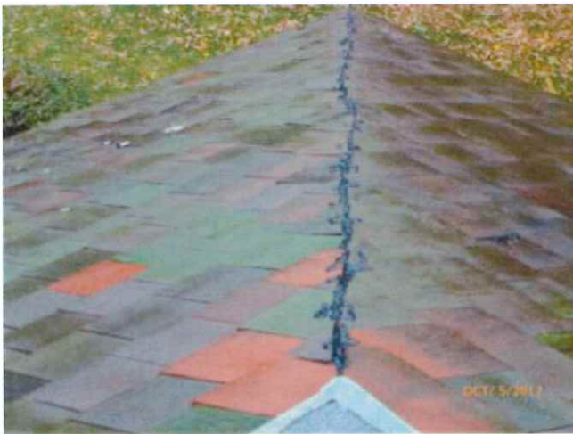
Missing tile ridge cap
