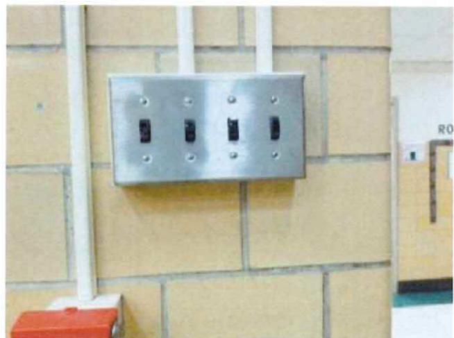
Student Dining Multilevel Switching
