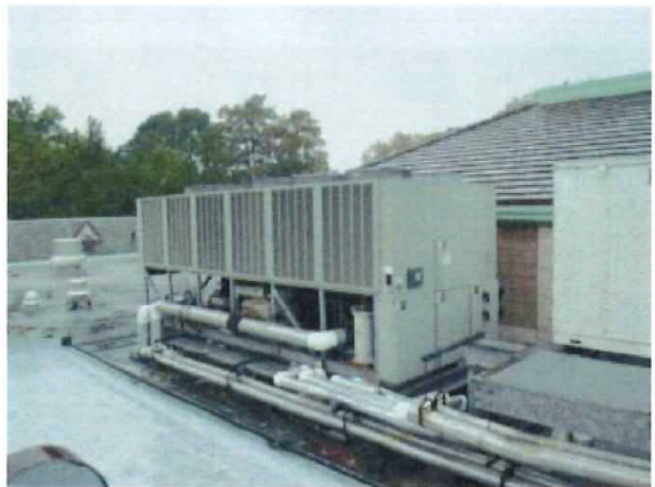
Air Cooled Chiller
