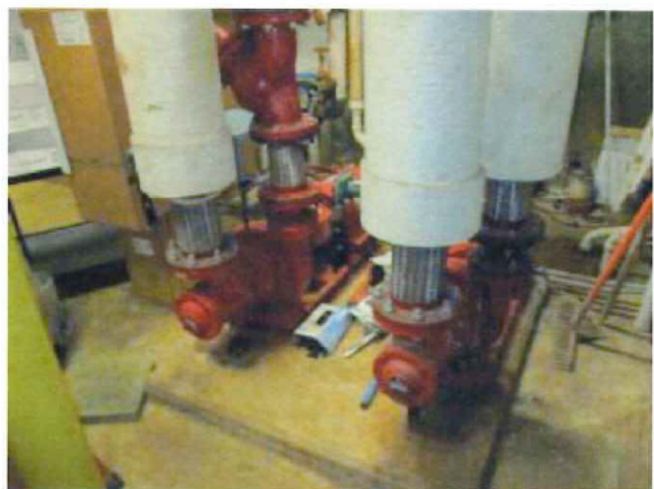
Heating Hot Water Pumps
