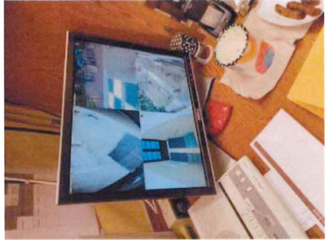
CCTV Monitor with All Zones Shown
