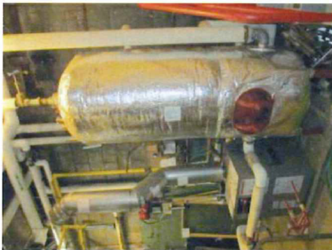
Gas Fired Water Heater
