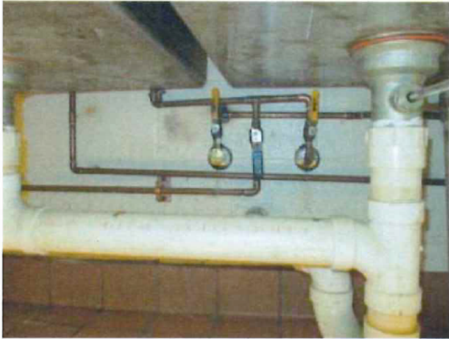
Kitchen Sink Waste
