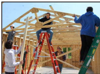
Students Construct Barn. Photographed in May 2023 by Beth Nash, BOCES 2 Communications Specialist.
