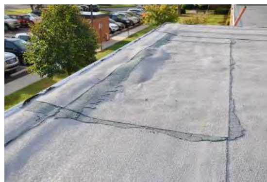
Top: Outdated HVAC Bottom: Timeworn Roof
