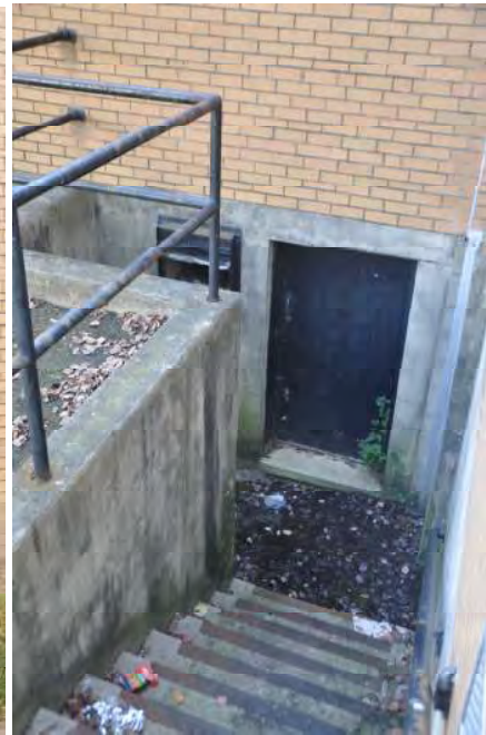
Inadequate drainage at stair well
