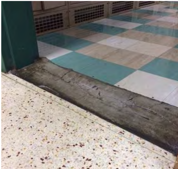
Differential floor elevation due to structural settlement
