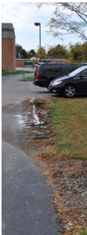
Site drainage issues
