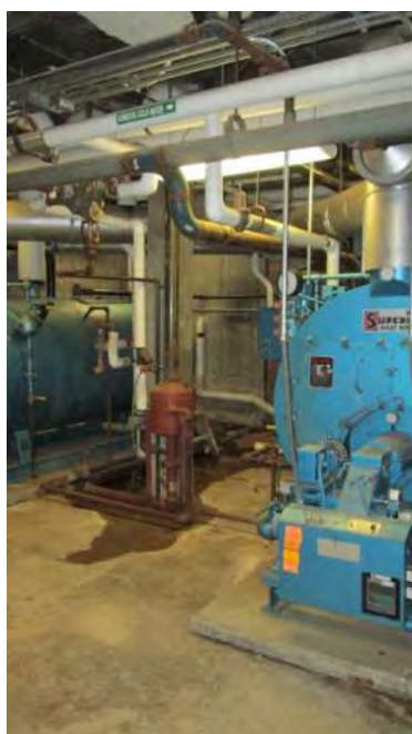
Outdated HVAC equipment
