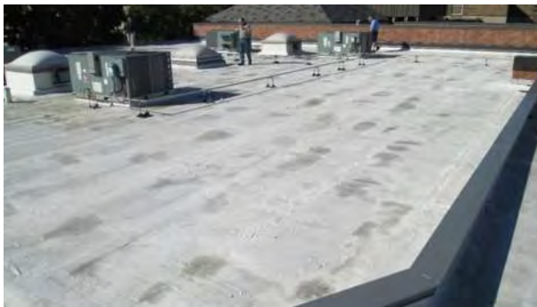
Roof sections in need of repair/replacement
