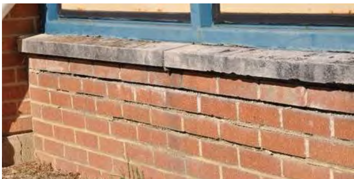
Top: Roof in need of repair Bottom: Failing exterior brick
