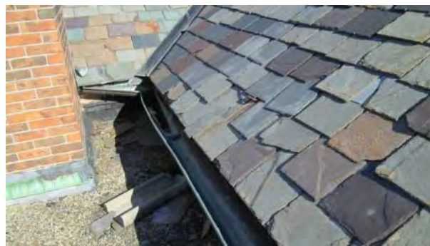
Damaged slate tile roof and drainage
