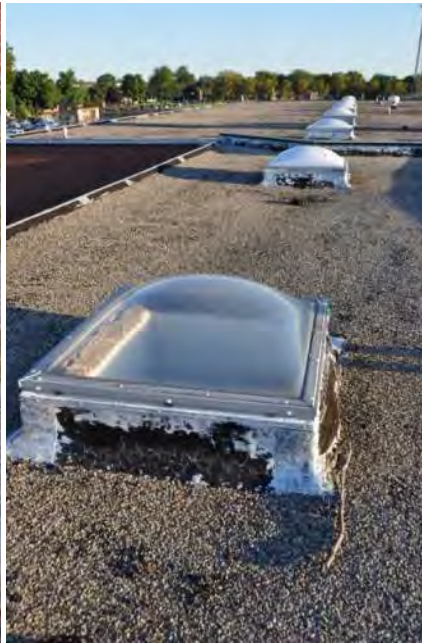
Roofing in need of repair
