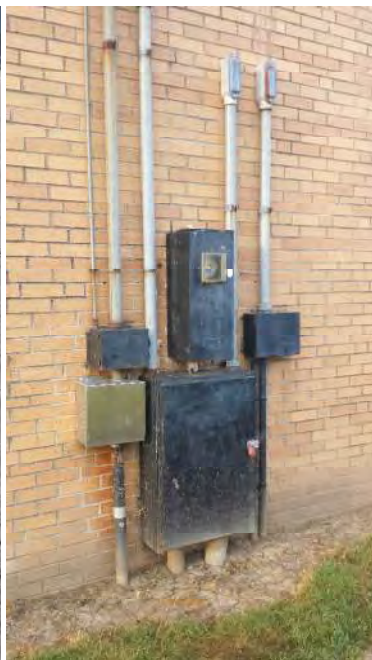
Outdated main electrical panel
