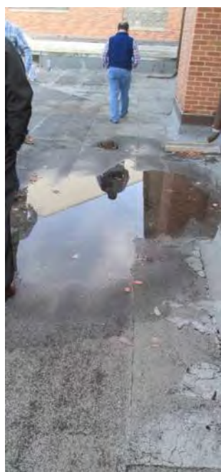
Roof needing repair
