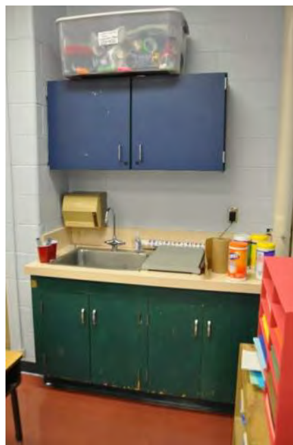
Casework in need of repair
