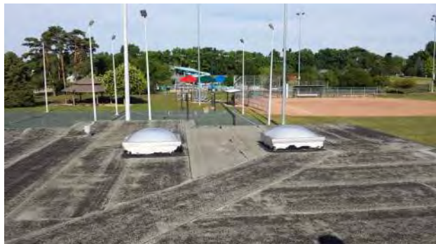
Roof sections in need of repair/replacement
