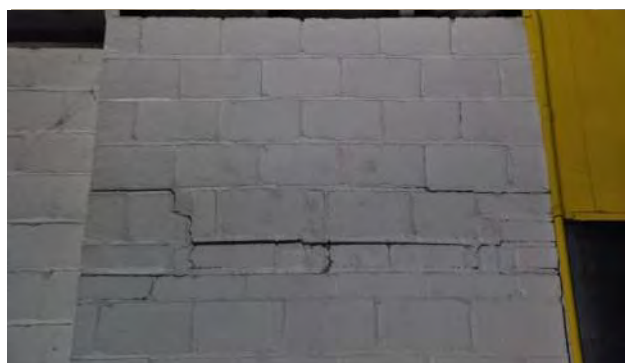
Masonry and structural settlement at Block House
