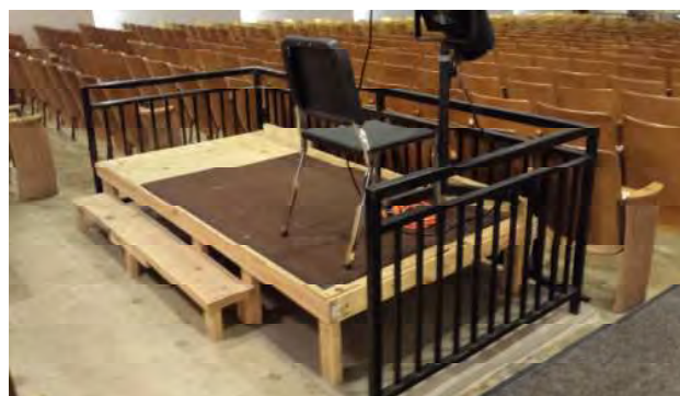
Auditorium finishes in need of repair/upgrade
