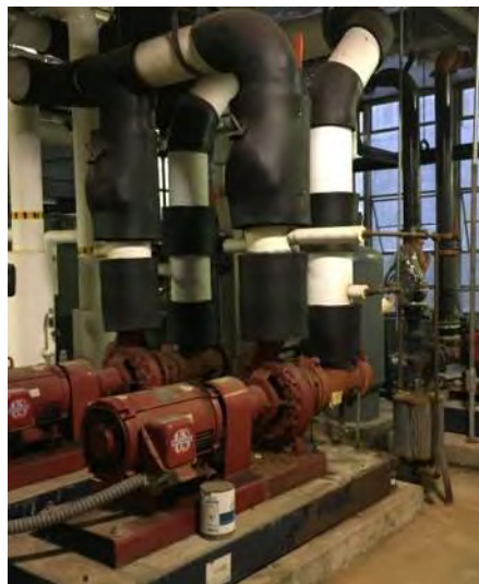
Dated HVAC systems
