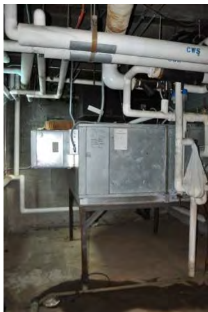
Timeworn HVAC system
