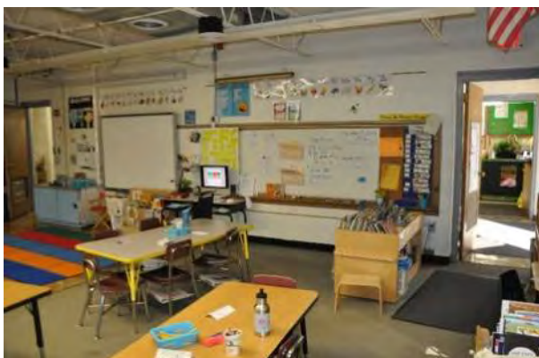
Classroom general finish upgrades needed
