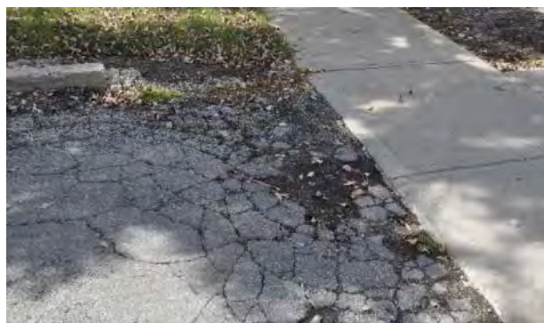
Asphalt damage at parking
