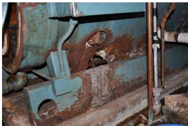
Failing HVAC specifically the existing boilers
