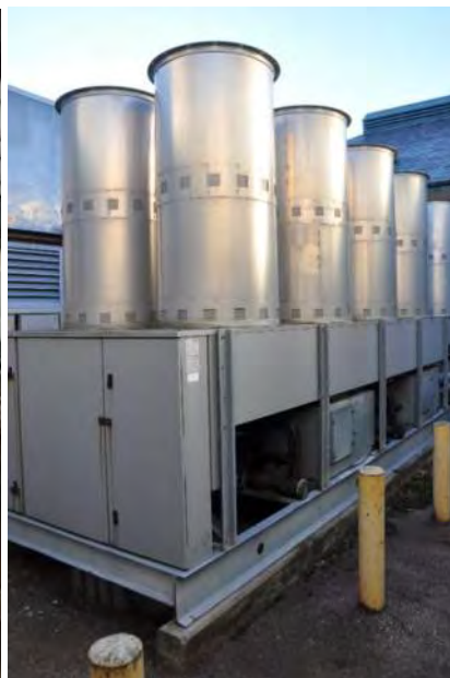
Building chiller near end of life
