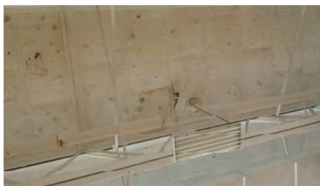
Gymnasium roof structure with water staining
