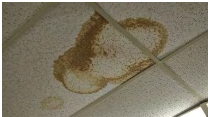
Water infiltration at floor and roof
