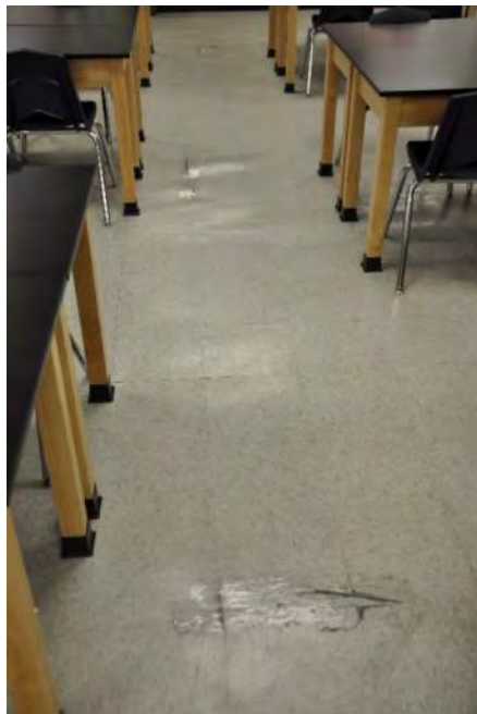
Damaged floor tiles
