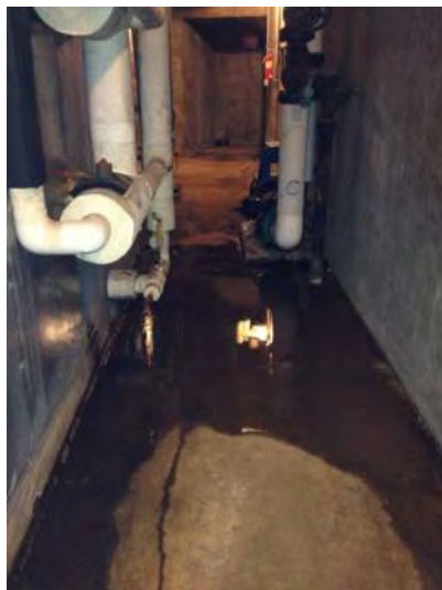
Basement Water Infiltration
