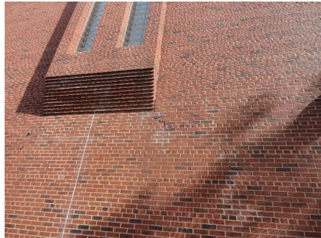
Brick wall crack at natatorium.
