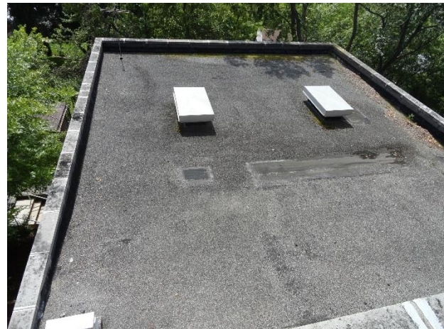
Roofing is in poor condition.
