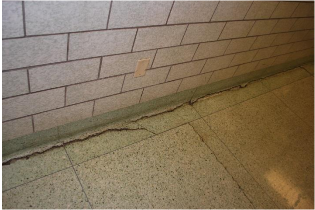
Terrazzo flooring is cracked at some locations.
