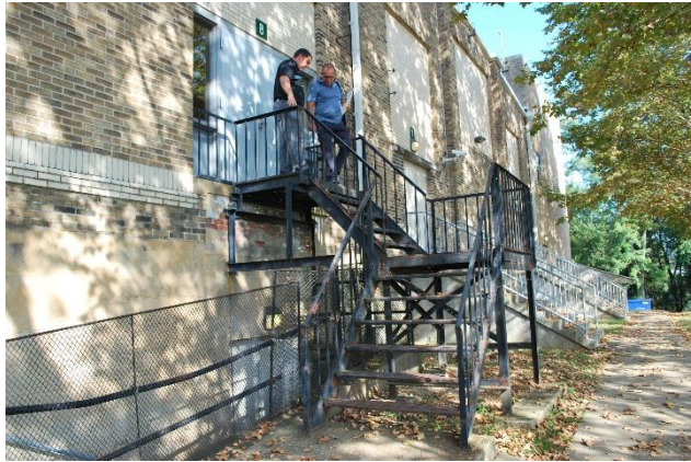
Emergency Exit Stairs leading to front sidewalk.
