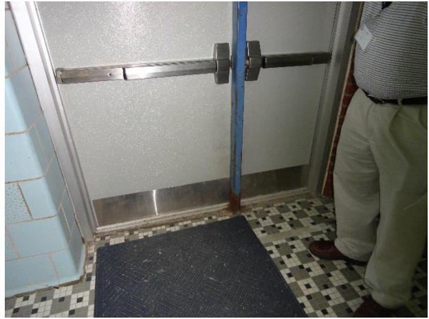
Natatorium: rusted exterior frames.
