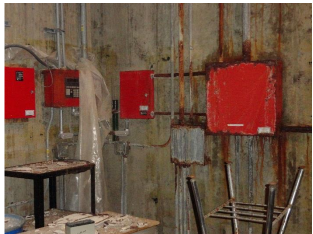
Corroded piping in basement.
