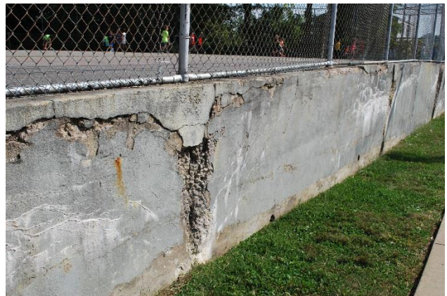
Another view of severely eroded playground retaining wall, located between playground and street.
