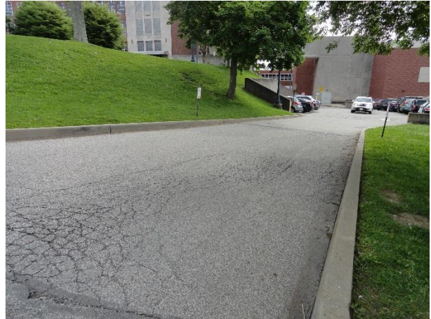
Paving is in poor condition.
