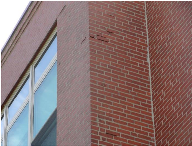
Typical exterior brick with some areas that need repairs.
