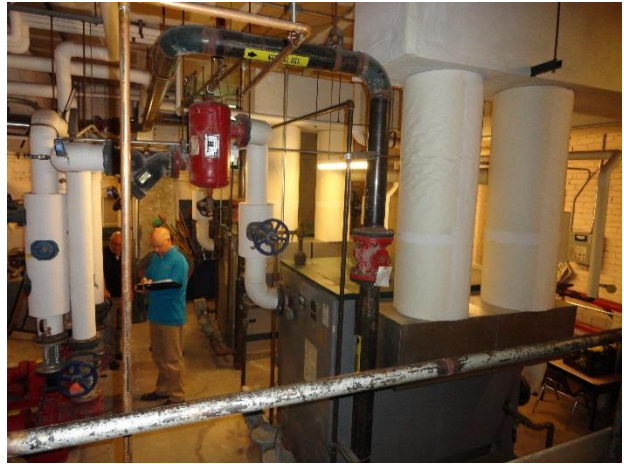
Mechanical space in basement.
