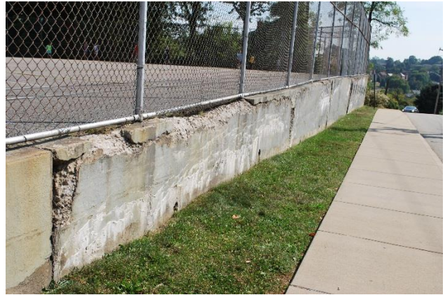
Severely eroded retaining wall between playground and street.
