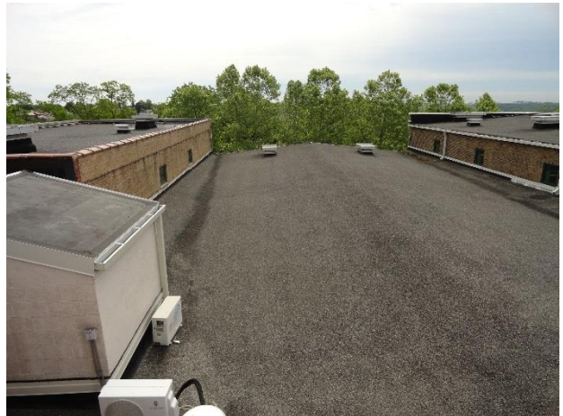
Roof is in poor condition.
