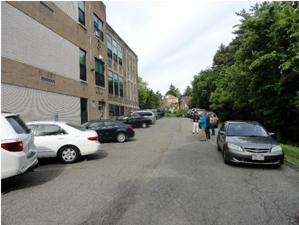
The paving is in poor condition and parking is inadequate.
