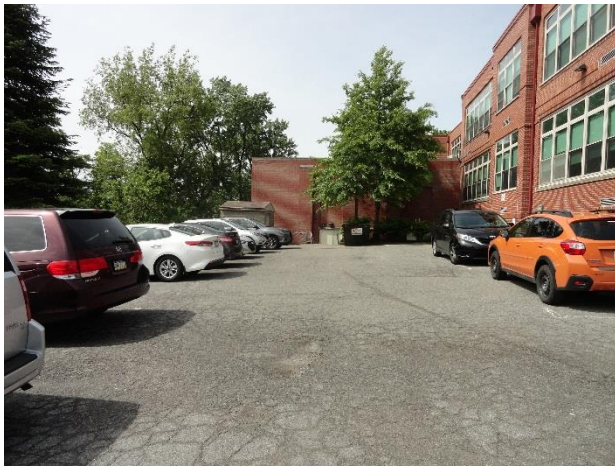
Exterior paving is in poor condition.
