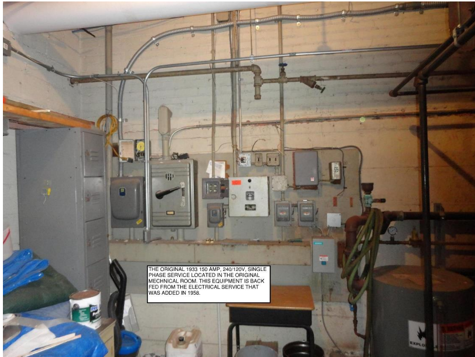
Original 1933 150-amp, 240/120-volt service, back fed from the 1958 service.
