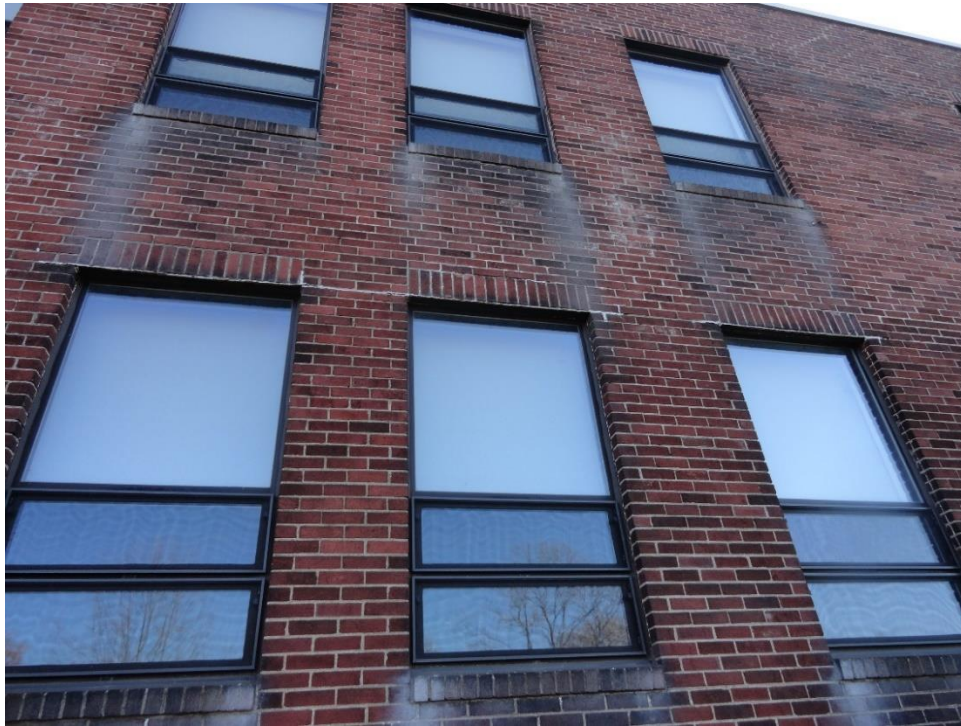
Exterior Brick and Lintels are in poor condition.
