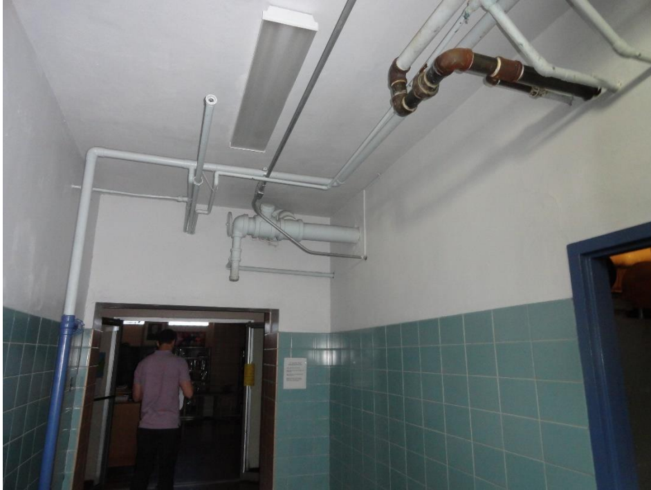
Antiquated Steam Heat Pipe System.
