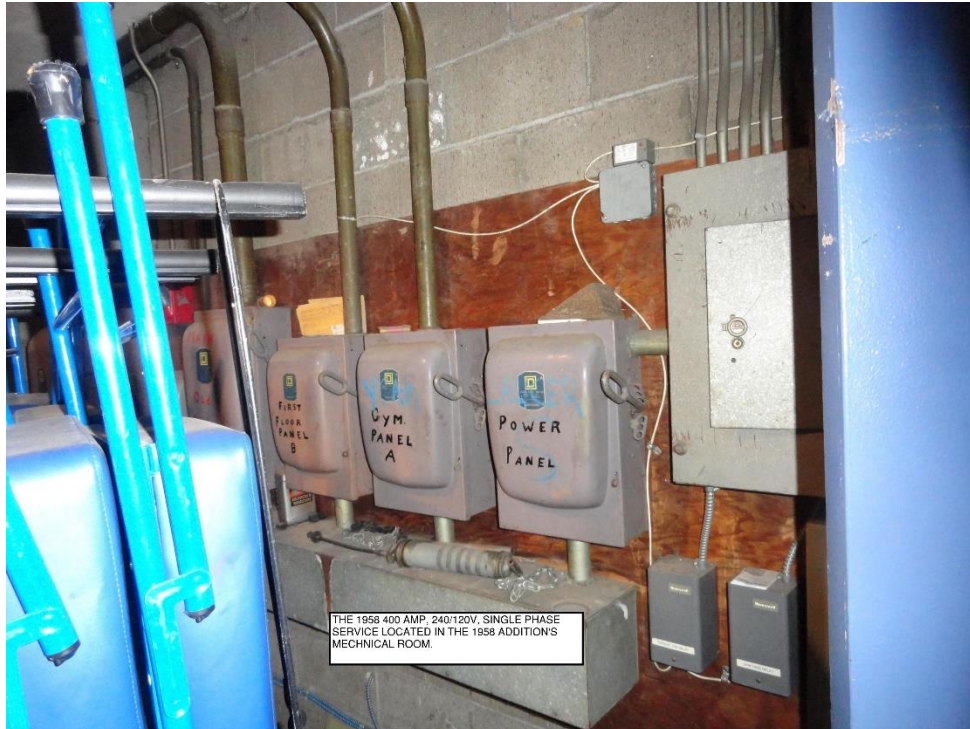
1958 400-amp 240/120-volt single phase service.
