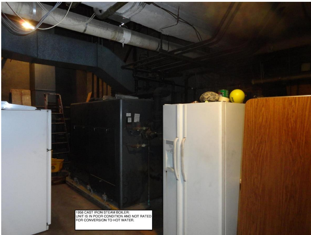
1958 cast-iron steam boiler is in poor condition and not rated for conversion to hot water.
