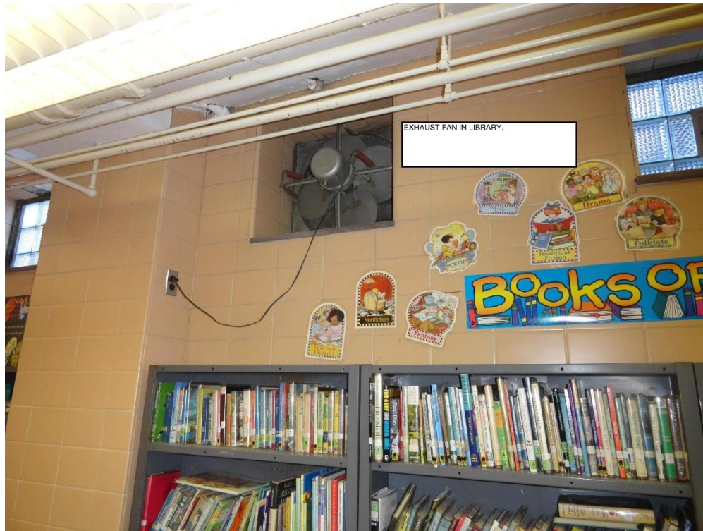
Exhaust fan in Library.
