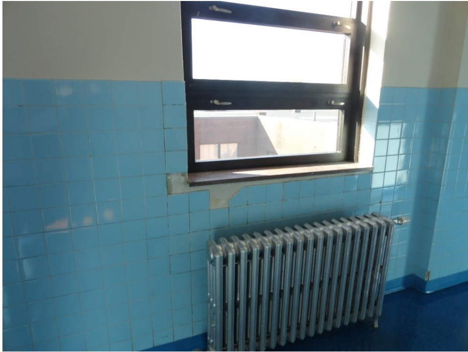
Hallway wall tiles are loose and missing.
