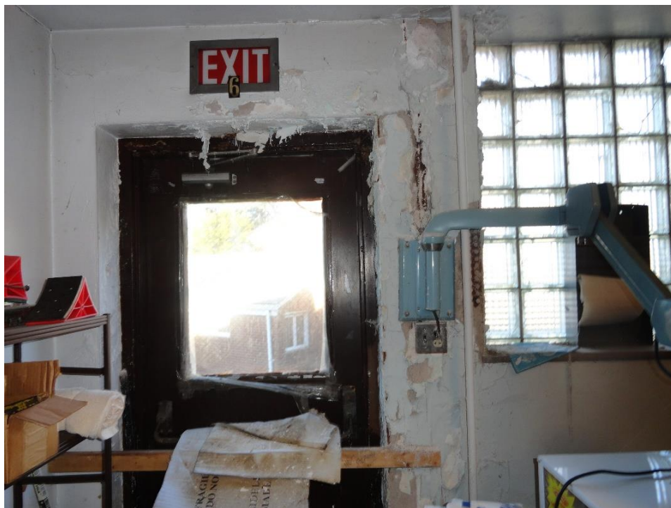
Lower level moisture intrusion damage.
