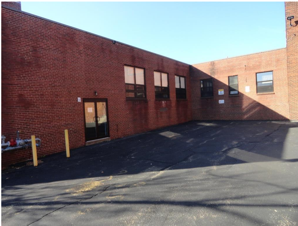
Asphalt is in poor condition.
