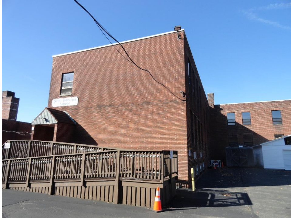
Handicap access ramp is in poor condition.
