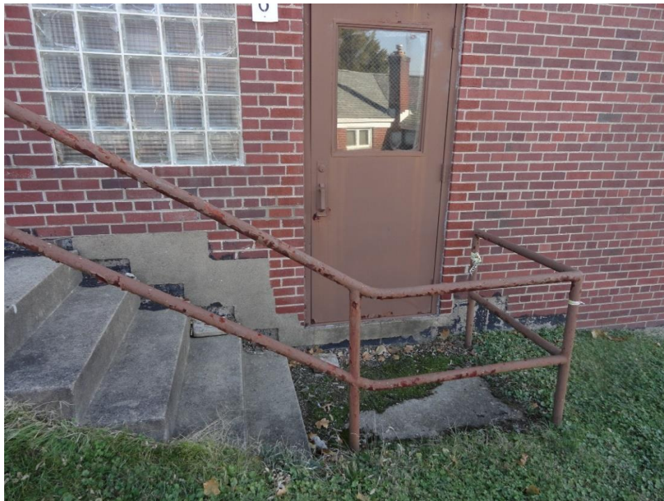
Exterior Concrete Steps and Landings are in poor condition.
