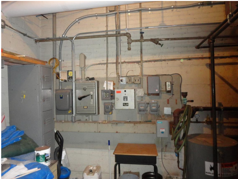
Inadequate & outdated Electrical System.
