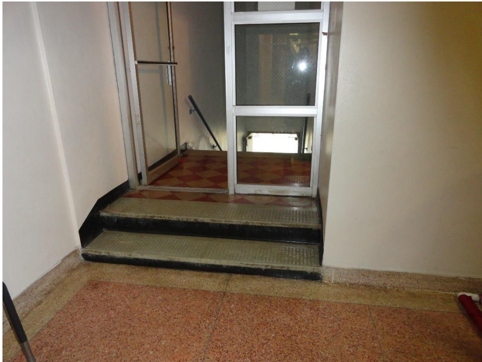
Non-standard, non-code compliant stair configurations.
