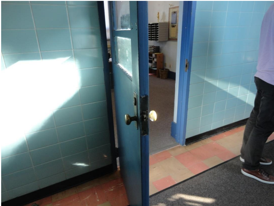
Interior doors are not ADA-compliant in many locations.
