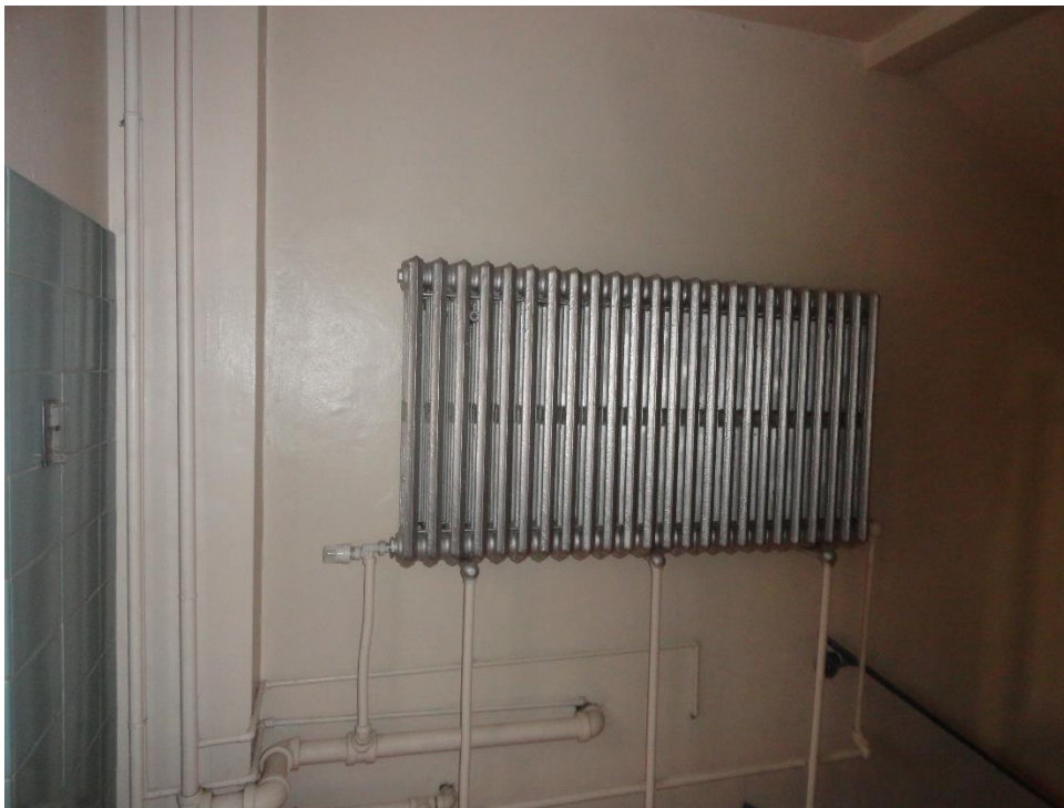
Exposed cast-iron steam radiators are original to the building.
