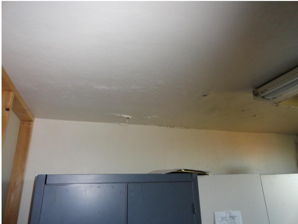
Upper level moisture intrusion damage.
