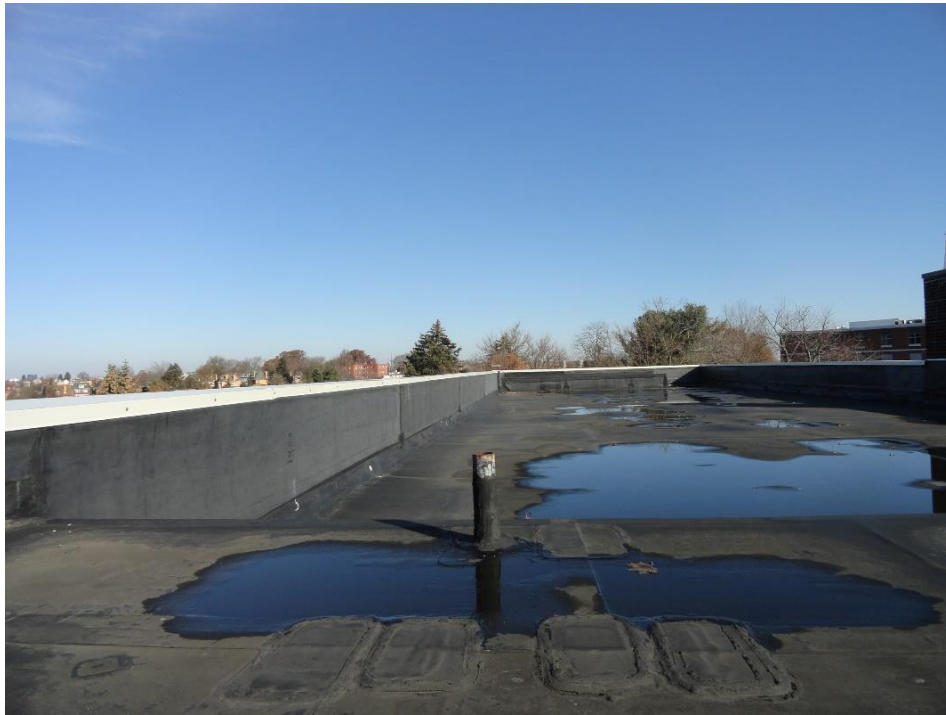
Aged EPDM rubber membrane and standing water.
