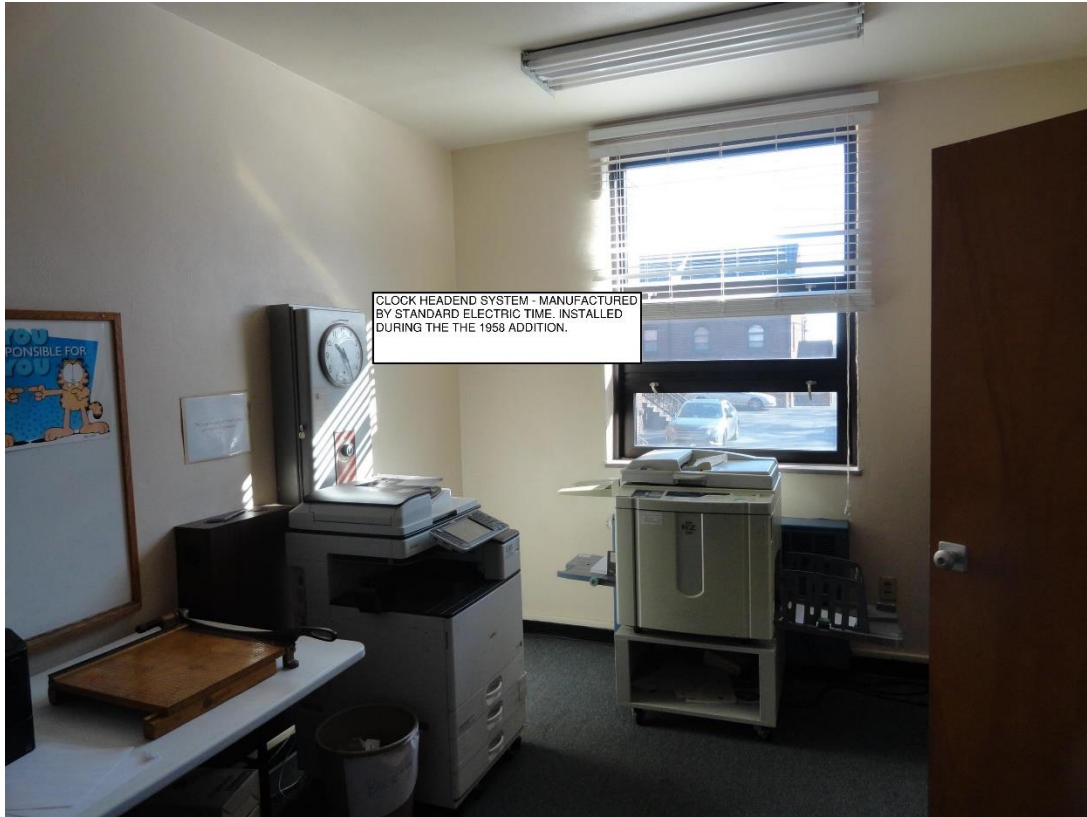
Clock head-end system installed in the 1958 addition.
