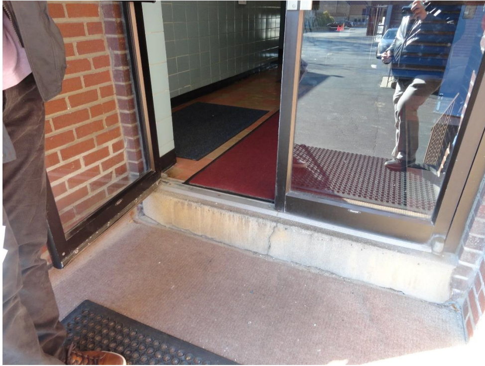
Non-code compliant riser at entry.
