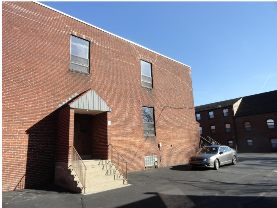
Building ADA access concerns.
