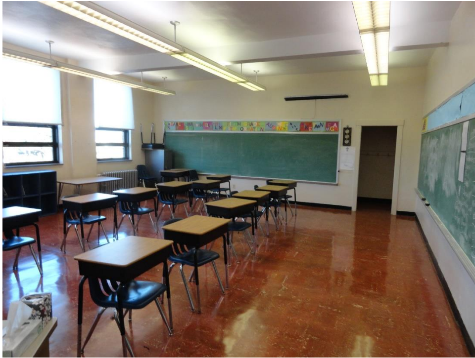
Likely Asbestos-containing floor tile throughout.
