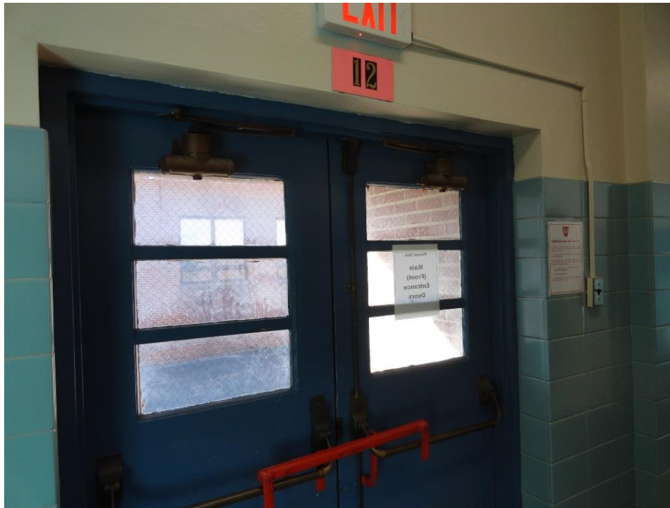
Exterior doors are not ADA-compliant in many locations.
