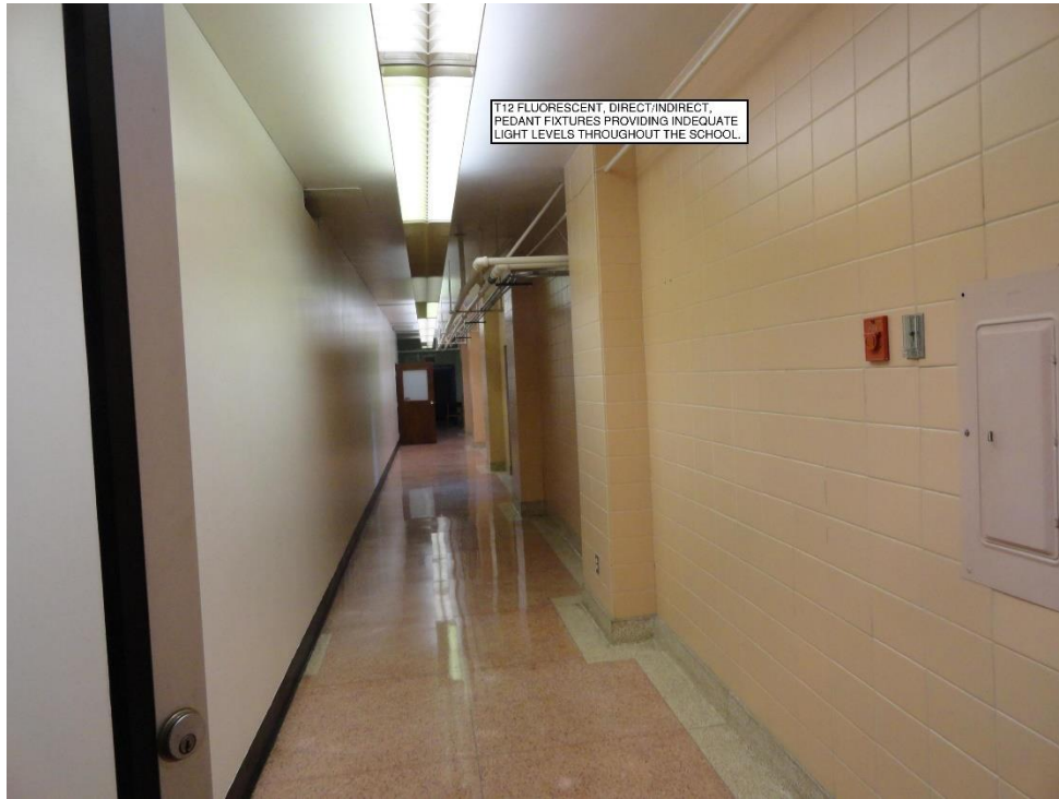
T12 Fluorescent lighting is providing inadequate lighting.
